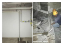
Plumbing and sanitary systems Supply and install water supply sanitary and drainage systems, cold water supply systems, sanitary systems and rainwater drainage systems
