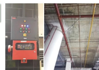
Fire protection systems Supply, install, test and commission of equipment, piping networks, appliances and fittings for fire protection systems
