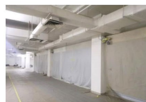
Air and mechanical ventilation (ACMV) systems Design, supply and install ACMV systems
